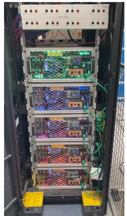
FIGURE 1 – Electrical cabinet with 10 opENS inverters.
